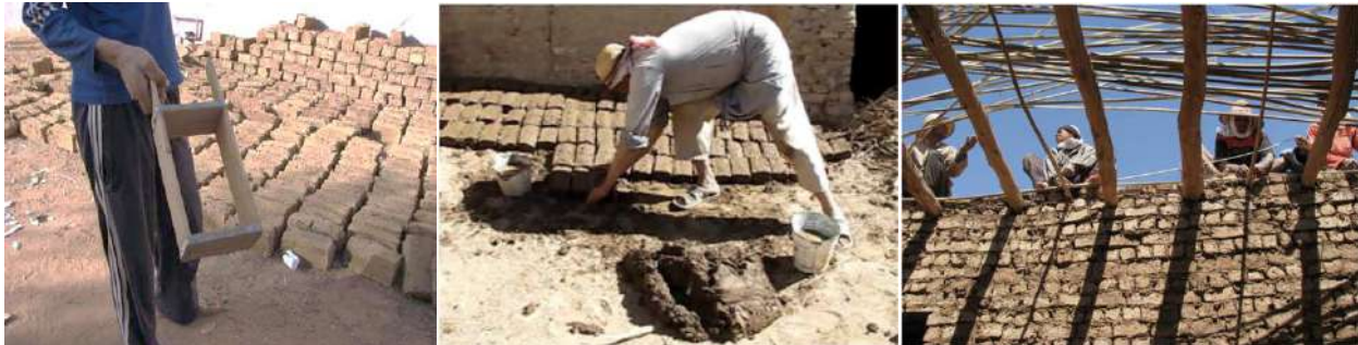
Figure 14: The usage of adobe clay bricks, together with reeds and acacia wood, in construction at Balat Town in El-Dakhla Oasis.
